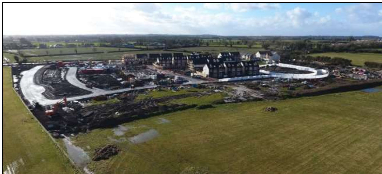
Figure 2.3: Phase 1A and 1B developments under construction to the south of the SHD site
